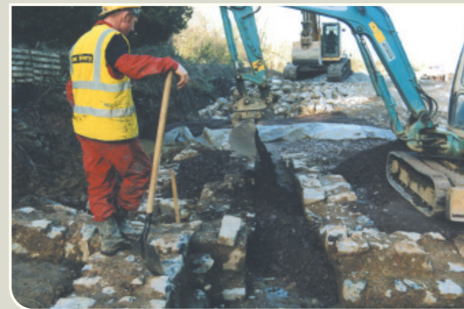
Works being carried out to ensure the preservation in situ of Ballyseedy mill . (Photo Eachtra Archaeological Projects Ltd.)
